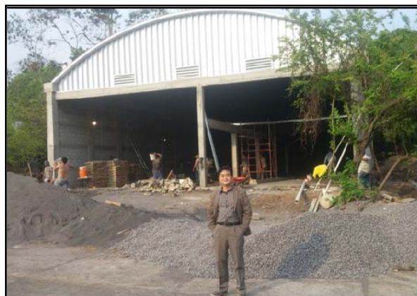
CFO Jong Myung (James) Choi outside the Sollen-Mobile Factory during Construction, March 2015
